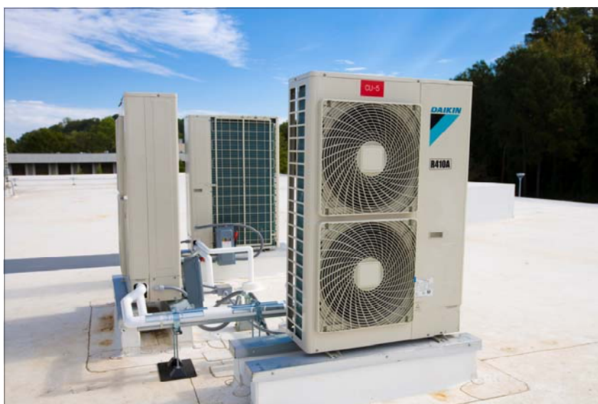
The HVAC system included a Daikin VRV ® -S Heat Pump System. Design and installation of the inverter-controlled systems was supported and serviced by Daikin during the project.
