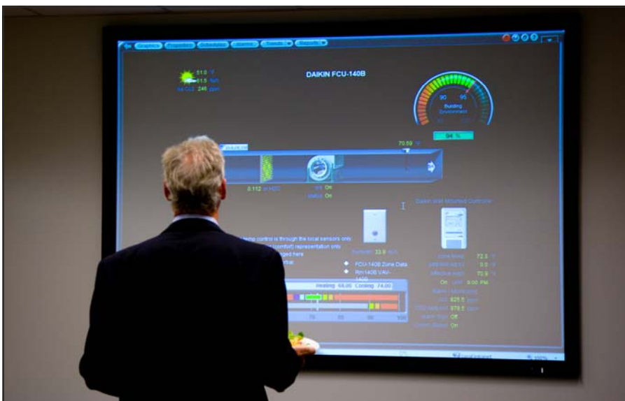
Daikin's equipment's performance can be monitored in real time throughout the building of ASHRAE's new sustainable headquarters.
