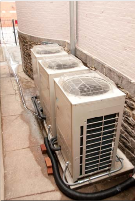
Daikin RXYQ outdoor condensing units at the rear of the synagogue which supply a total of 28 tons of capacity.
